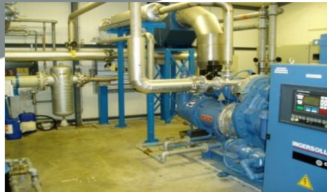
High Pressure Air Plant
