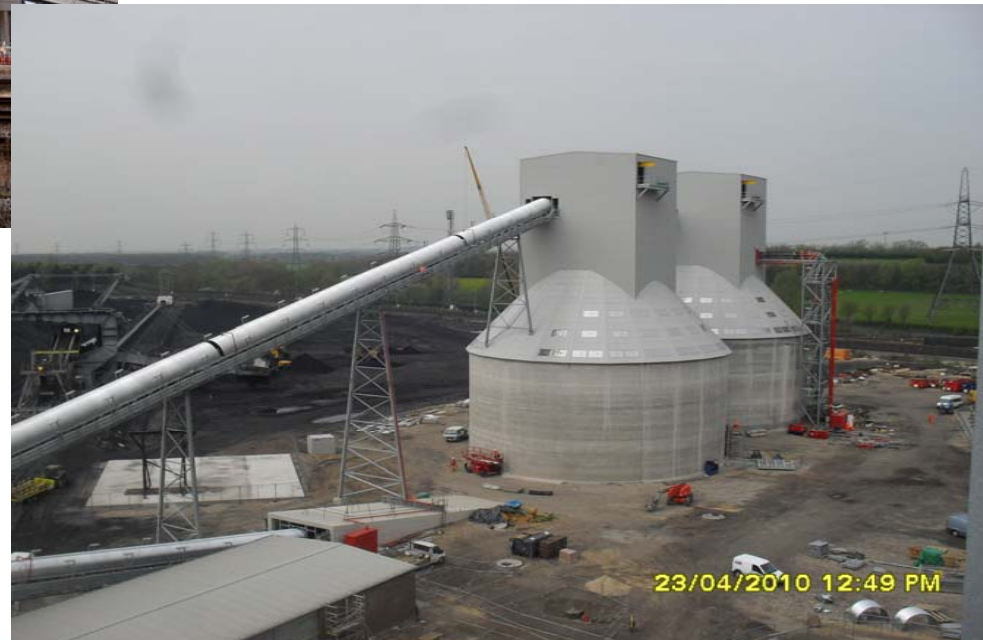
Rail storage 16,500 tonnes
